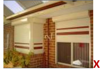
NON-COMPLIANT ROLLER SHUTTERS
